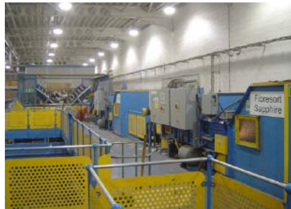
Typical MRF sorting facility
